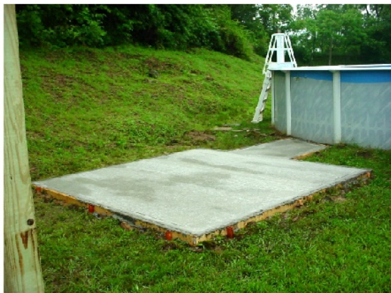
In between the rain we were able to pour concrete for the footers for one project and had enough concrete to pour a new "Foursquare" game area.
