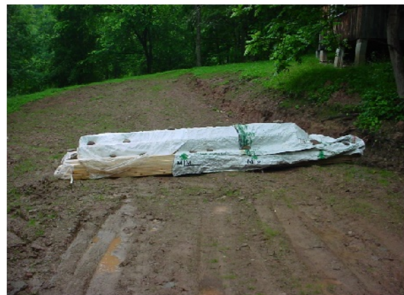
Some of the building materials for the "Campfire Building" waiting and covered over to protect from the rain.
